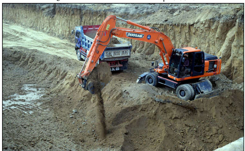
ISLAMABAD: Heavy machinery in action for the construction of 9th Avenue F-9 underpass and flyover project in the Federal Capital.
