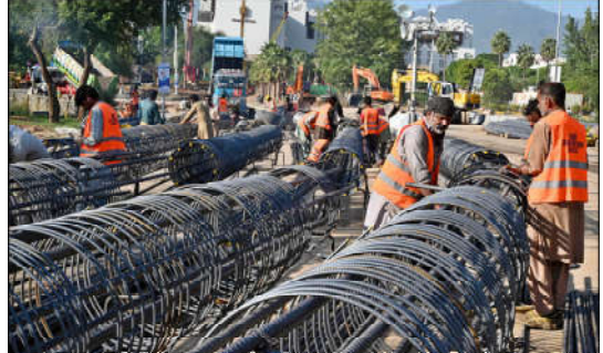
ISLAMABAD: Laborers are busy binding steel at the construction site of an underpass along Khyaban-e-Suharwardi in the Federal Capital as part of ongoing development work.
