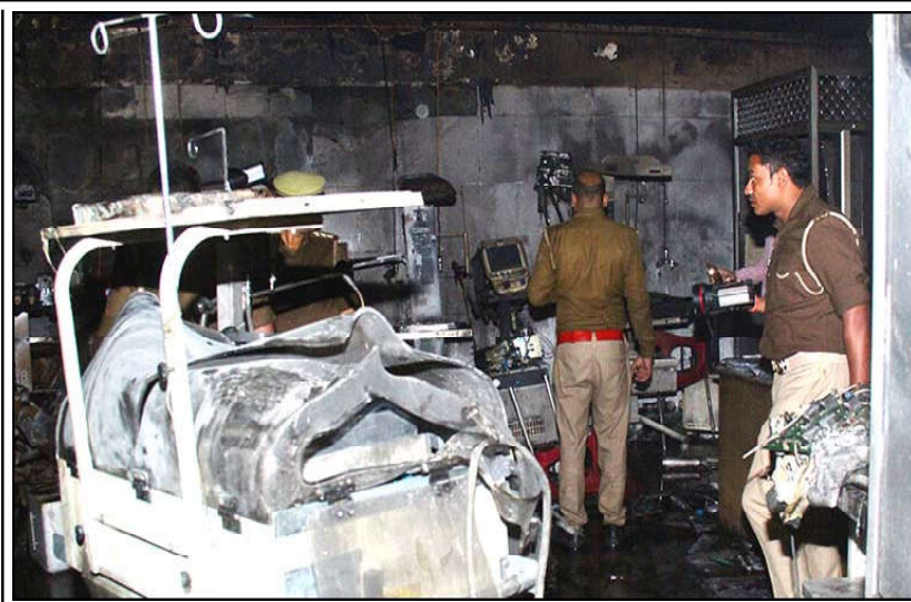
Police officers examine the damaged neonatal intensive care unit after a fire broke out at the Maharani Laxmibai Medical College in Jhansi district, in the northern state of Uttar Pradesh, India.
