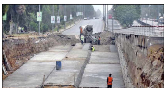
ISLAMABAD: A development project is underway as heavy machinery is being used in the construction work at the PTCL Chowk Underpass, aimed at improving traffic flow and infrastructure in the heart of the Federal Capital.
