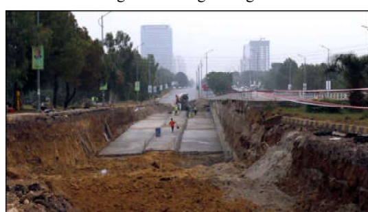
ISLAMABAD: A major road network project is underway at the PTCL Chowk underpass in the heart of the capital, aimed at improving traffic flow and enhancing infrastructure.
