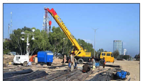
ISLAMABAD: Heavy machinery being used at the site of under-construction PTCL Chowk underpass project during development work in Federal Capital.
