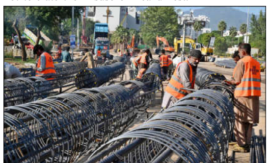
ISLAMABAD: Laborers are busy binding steel at the construction site of an underpass along Khyaban-e-Suharwardi in the Federal Capital as part of ongoing development work.
