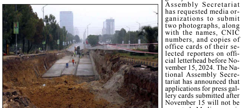
ISLAMABAD: A major road network project is underway at the PTCL Chowk underpass in the heart of the capital, aimed at improving traffic flow and enhancing infrastructure.
