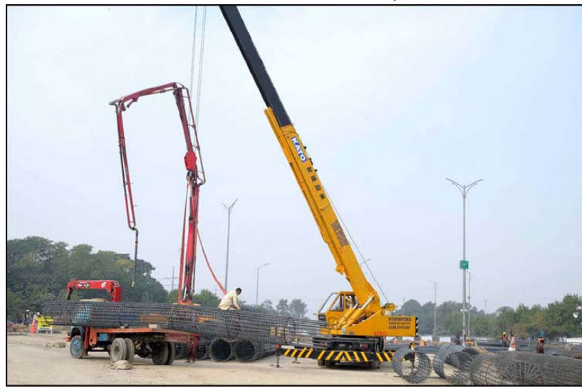
ISLAMABAD: Heavy machinery being used at the site of under-construction PTCL Chowk underpass project during development work in Federal Capital.
