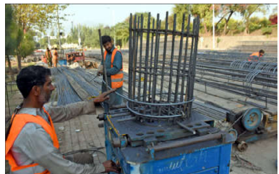
ISLAMABAD: Laborers are busy in laying the foundation of pillars during the construction work of interchange at Sarena chowk as this is the project of CDA following the mission of Make the Capital beautiful.
