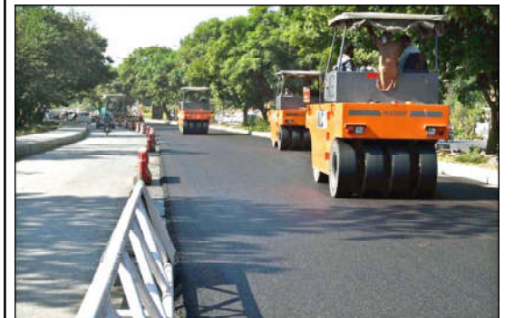
ISLAMABAD: Heavy machinery being used during extension work of Club Road during development work in Federal Capital.
