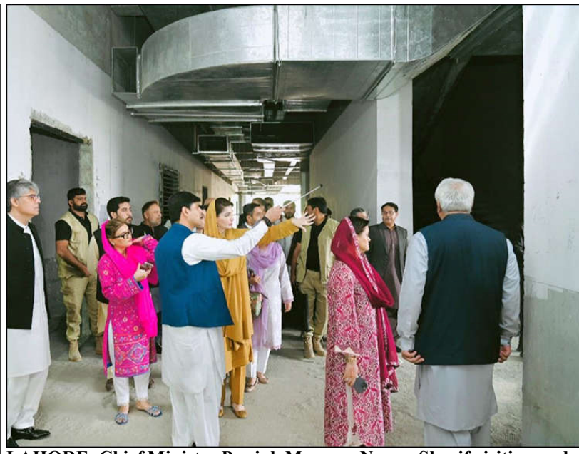
LAHORE: Chief Minister Punjab Maryam Nawaz Sharif visiting under construction Punjab Institute of Cardiology-II (PIC-II) at Canal Bank.
