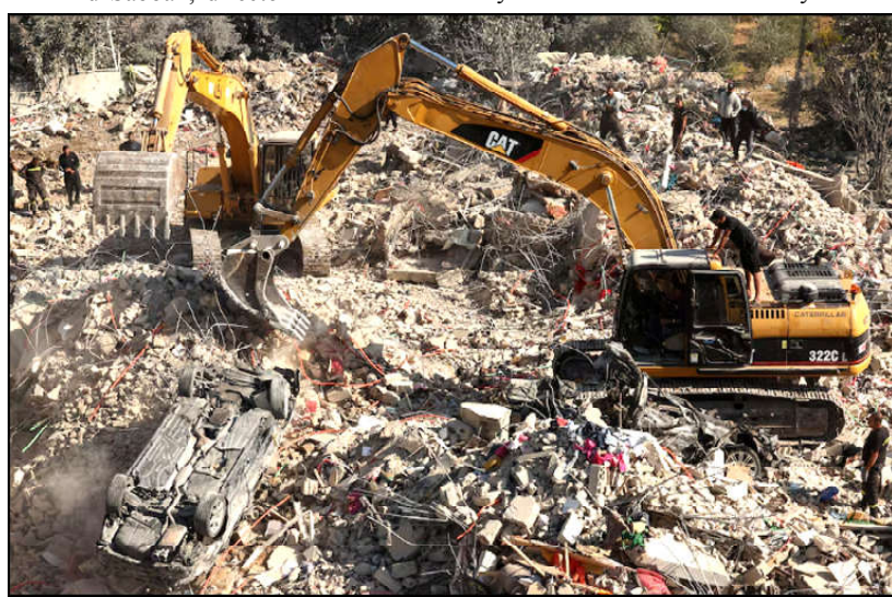
Excavators operate at the site of an Israeli strike, amid ongoing hostilities between Hezbollah and Israeli forces, in the southern Lebanese town of Sarafand, Lebanon.
