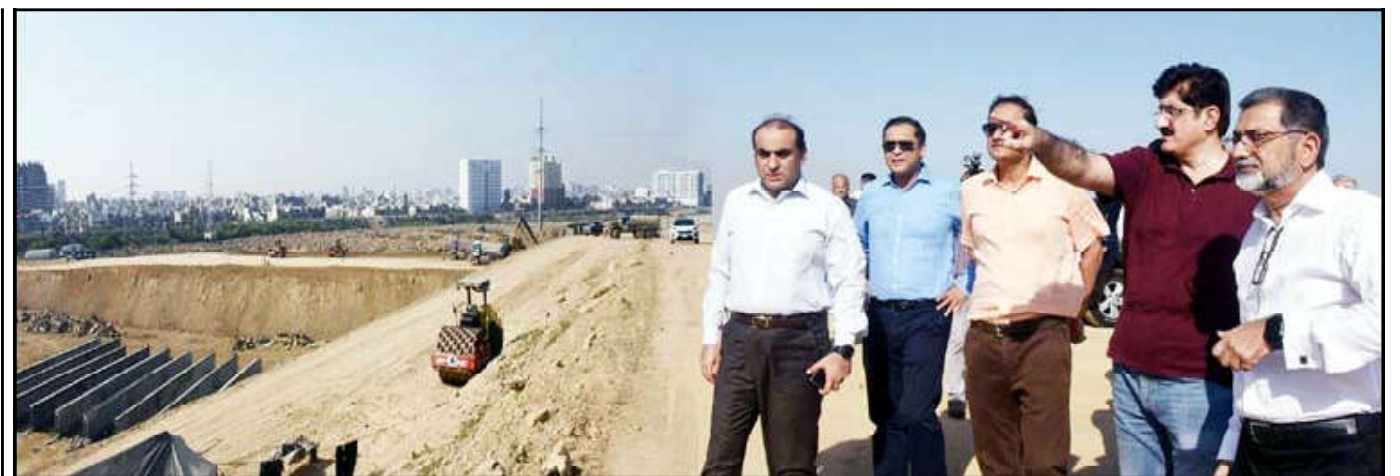
KARACHI: Sindh Chief Minister, Syed Murad Ali Shah inspects the progress and quality of the construction work of Malir Expressway, in Karachi.
