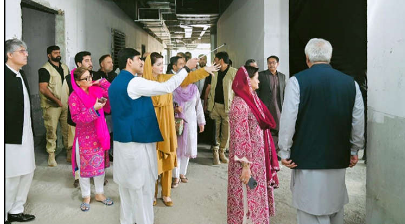
LAHORE: Chief Minister Punjab Maryam Nawaz Sharif visiting under construction Punjab Institute of Cardiology-II (PIC-II) at Canal Bank.
