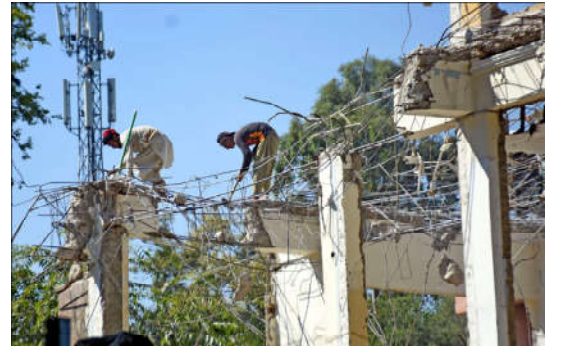
ISLAMABAD: Laborers are busy in dismantling a building at Sitara Market in the Federal Capital.
