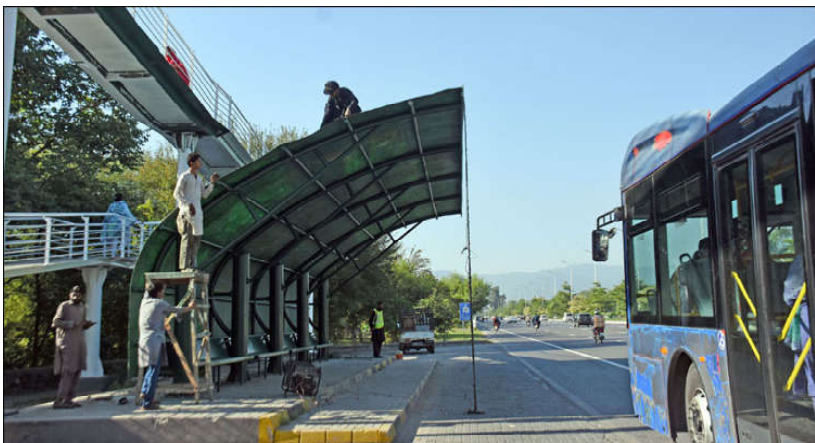
ISLAMABAD: CDA workers repairing a bus stop at Islamabad Expressway in the Federal Capital.
