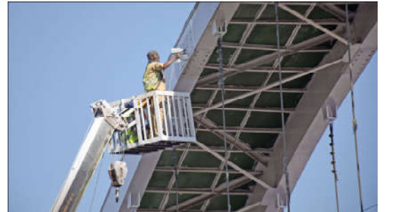
ISLAMABAD: CDA staff busy in the maintenance work of an overhead bridge.
