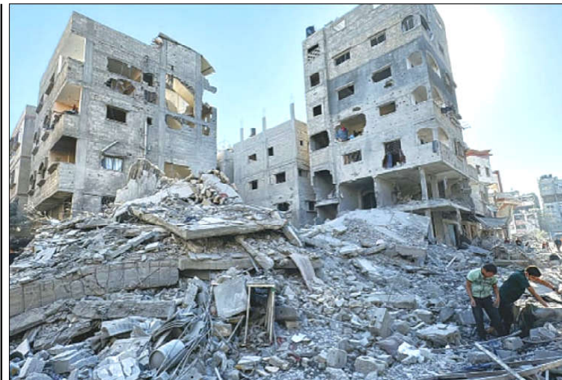
Palestinians inspect the damage after an Israeli air strike at Beit Lahya in the northern Gaza Strip.
