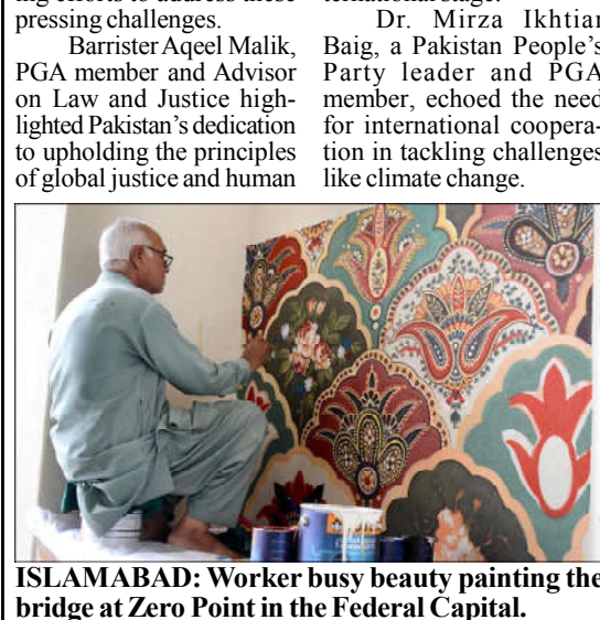
ISLAMABAD: Worker busy beauty painting the bridge at Zero Point in the Federal Capital.
