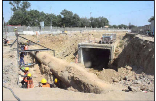
KARACHI: A view of ongoing construction work at the Numaish Chowranghi underpass in the provincial capital, aiming to improve city infrastructure.
