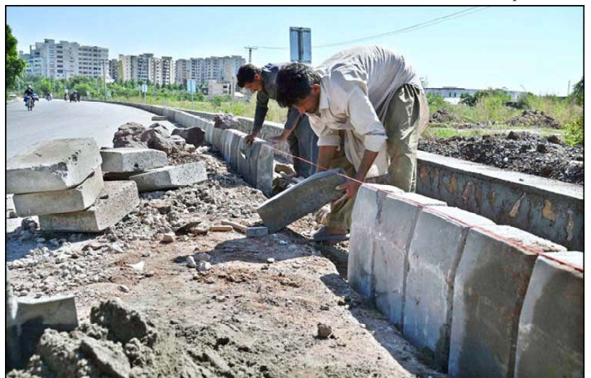
ISLAMABAD: Labourers busy in fixing cemented blocks along Club Road in Federal Capital.
