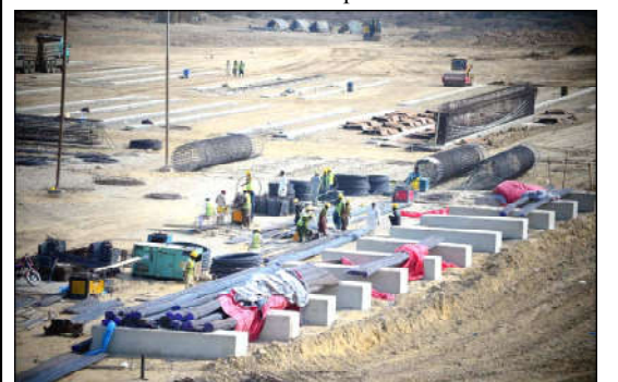
KARACHI: Construction works of Malir Expressway Korangi to Quaidabad Segment is underway under the supervision of local government department, at Korangi Industrial area in Karachi.
