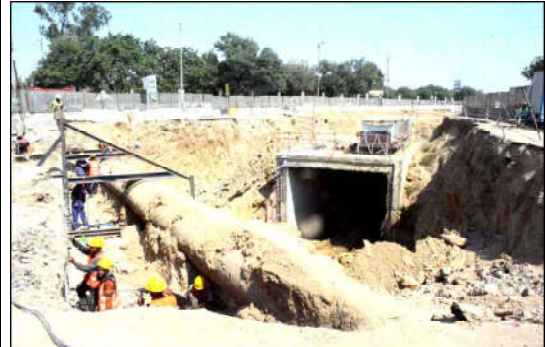
KARACHI: A view of ongoing construction work at the Numaiish Chowranghi underpass in the provincial capital, aiming to improve city infrastructure.
