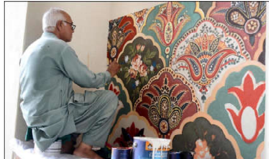
ISLAMABAD: Worker busy beauty painting the bridge at Zero Point in the Federal Capital.
