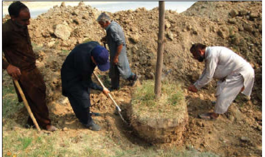
ISLAMABAD: CDA workers starts relocate the plants from the site of new flyover site on Jinnah Avenue.
