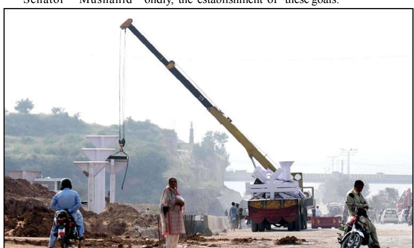
ISLAMABAD: Heavy machinery being used to install a pedestrian bridge on Islamabad Expressway.
