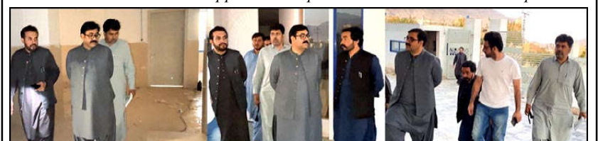
QUETTA: Provincial Health Minister Bakht Muhammad Kakar visiting different blocks during his visit to under construction Bacha Khan Hospital Nawan Killi.
