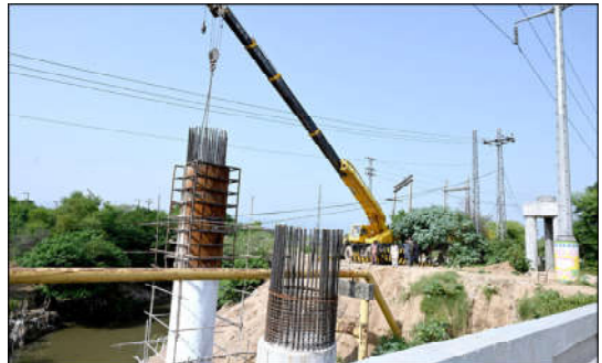
ISLAMABAD: Labourers busy in work of flyover under construction 10th Avenue during development work in Federal Capital.
