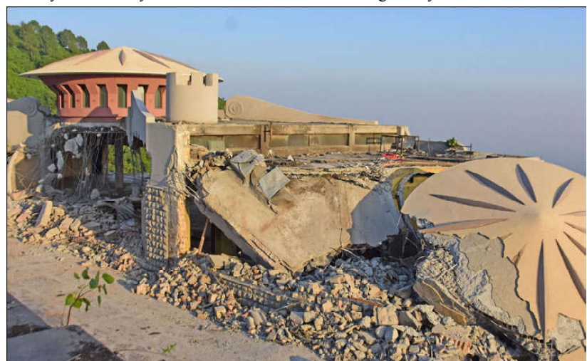
ISLAMABAD: Work in progress on Demolition of illegal constructions in Margallah Hills by Islamabad Wildlife Management Board.
