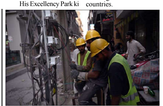
ISLAMABAD: IESCO workers install new Advanced Metering Infrastructure (AMI), driving innovation in the energy sector.
