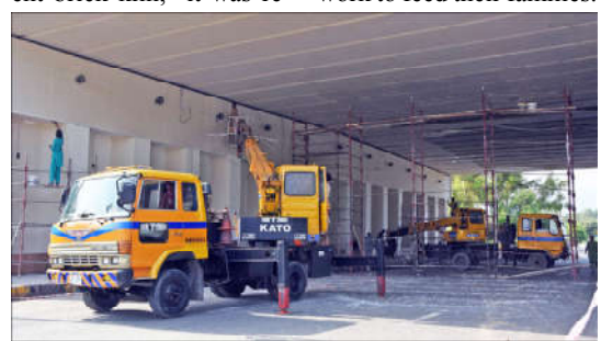
ISLAMABAD: Workers of Capital Development Authority (CDA) installing new colorful lights under zero point bridge, in the Federal Capital.
