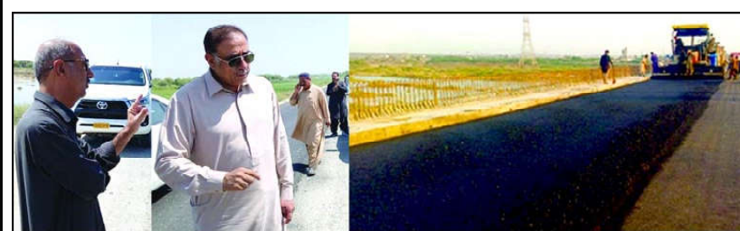
SOHBATPUR: Provincial Minister for Communication and Works Mir Saleem Ahmed Khosa inspecting under construction road from Sohbatpur to Kashmir
