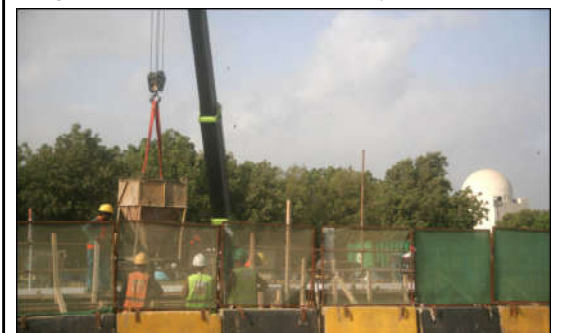
KARACHI: The construction work of Red Line Bus Service is in progress in front of Mazar Quaid, in the Provincial Capital.
