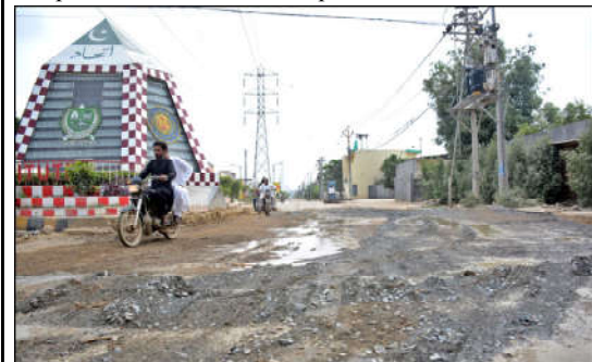
KARACHI: Roads leading to the Korangi Industrial Zone in urgent need of repair due to severe damage.
