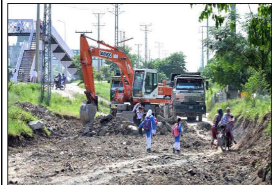
ISLAMABAD: Heavy machinery being used for the repair of Pandora Link Road in the Federal Capital.
