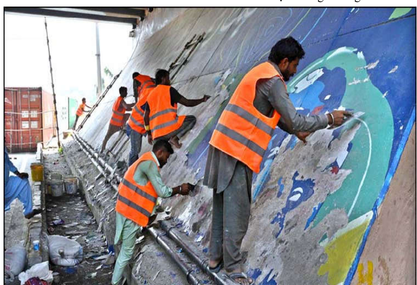
ISLAMABAD: Labourers are busy cleaning and removing old paint to repaint the wall under the Faizabad Interchange.
