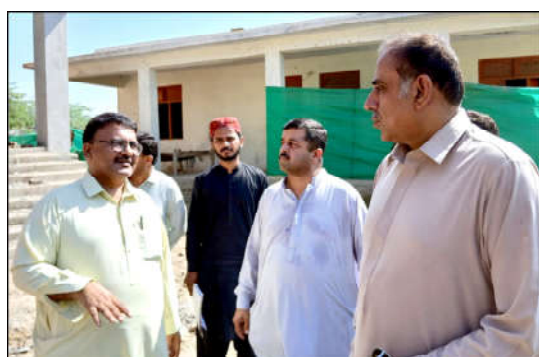
SOHBATPUR: Provincial Minister for Communication & Works Mir Saleem Khosa inspecting different development projects during his visit of Sohbatur.
