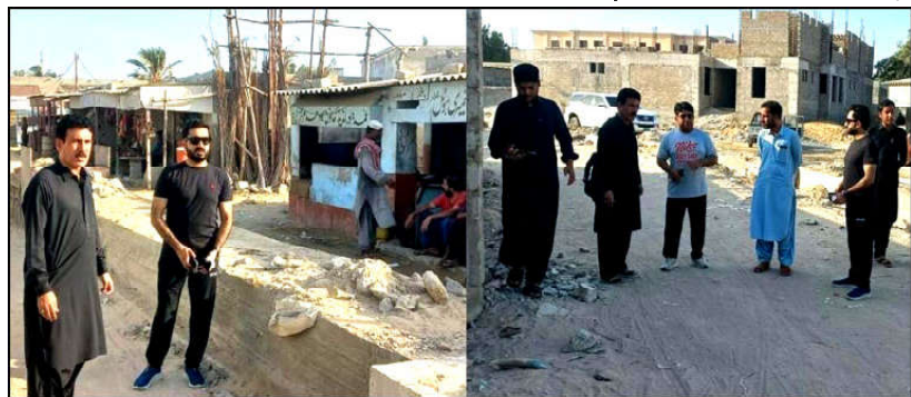
GWADAR: Director General GDA Shafqat Anwar Shahwani alongwith Assistant Commissioner Mir Jawad Ahmed Zehri inspecting under construction sewerage line project under Master Plan
