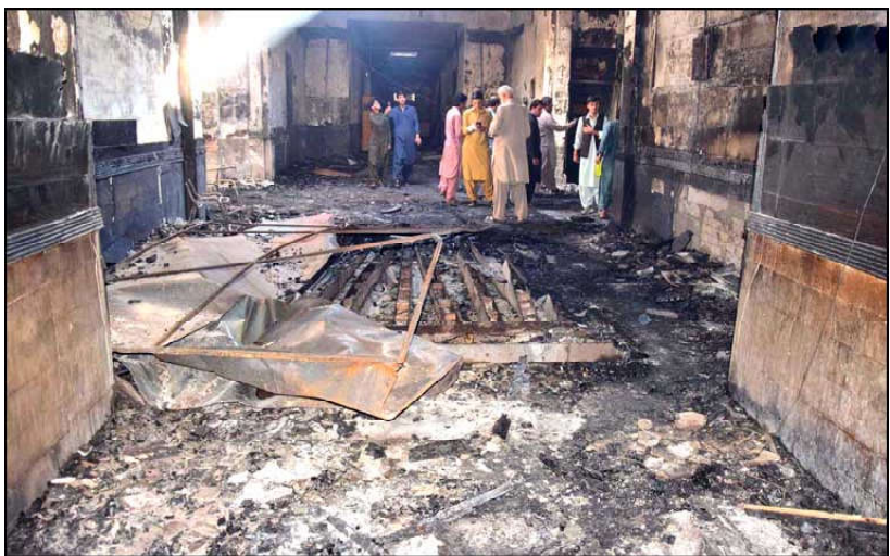
QUETTA: A view of damages due to fire at Science College
