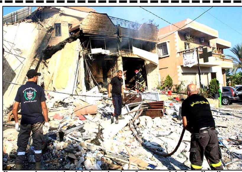
Rescuers inspect the debris at the site of an overnight Israeli strike on a pharmacy in the southern Lebanese village of Akbiyeh.
