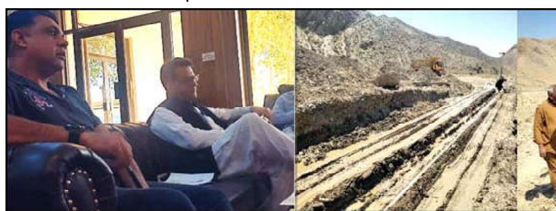
CHAMAN: Chairman Pakistan Railways and Federal Secretary Syed Mazhar Ali Shah inspecting the construction work of Khojak Tunnel and Railway track affected due to heavy rain and flood.
