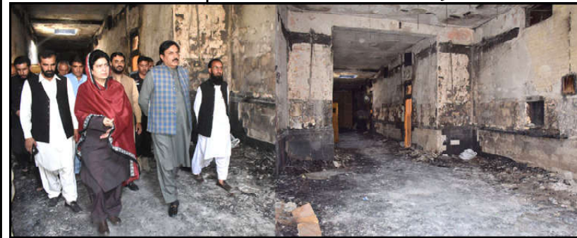
QUETTA: Deputy Chairman Senate Seydal Khan Nasar alongwith Provincial Minister for Education Raheel Durrani inspecting the burnt building of Govt Science College.
