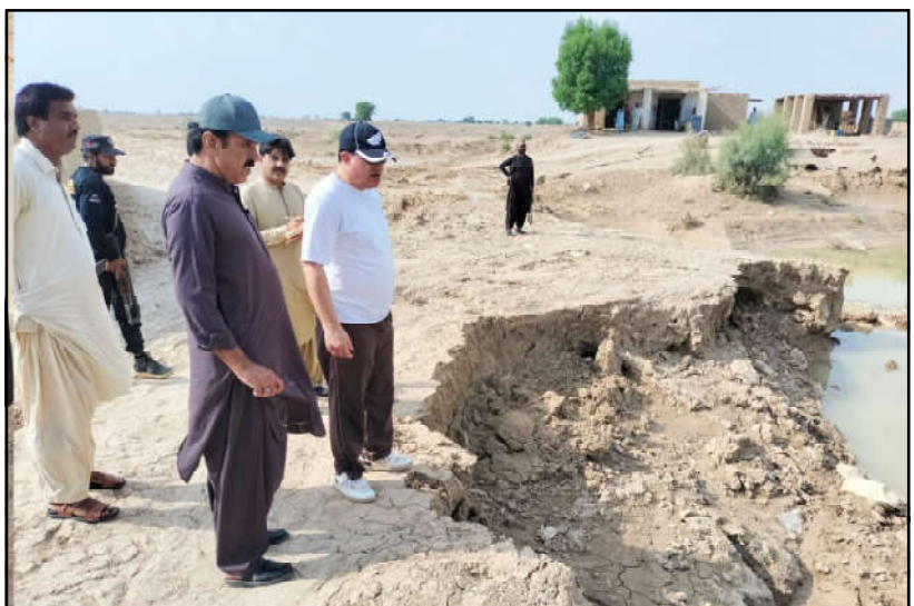
NASEERABAD: Deputy Commissioner Munir Ahmed Kakar being briefed by SDO Amanullah Gajani about crack in Rabi canal
