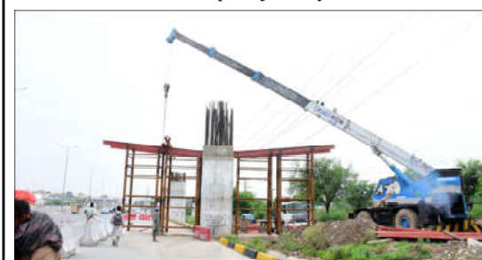
ISLAMABAD: Work in progress on a construction project at Karnal Sher Khan Road in the Federal Capital.
