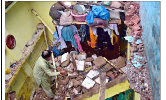
HYDERABAD: A view of the roof of a house collapsed due to heavy rain in the Old Vegetable Market area, resulting in the death of one child and injuries to four people.
