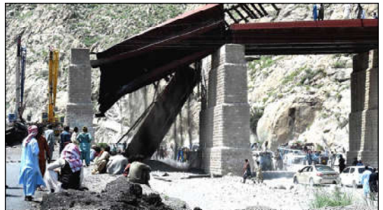
QUETTA: A view of labour busy in work on destroys Railway Bridge.
