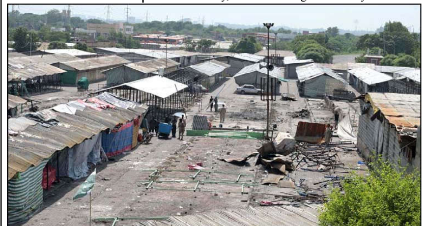
ISLAMABAD: A view of the workers busy rebuilding the stalls at the Peshawar Mor Weekly Bazaar, which was damaged due to a fire.
