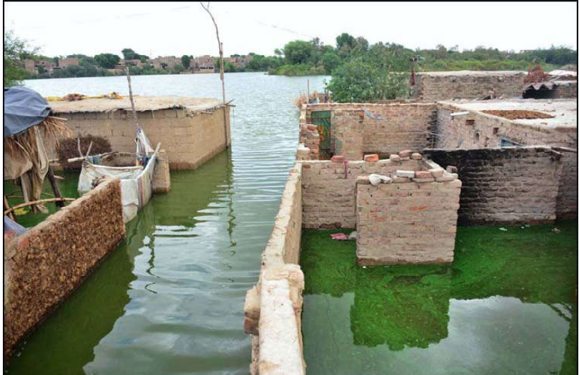
HYDERABAD: Residents of Saharash Nagar flooded, near the Indus River, as river waters overflow into homes, causing significant damage and widespread inundation.
