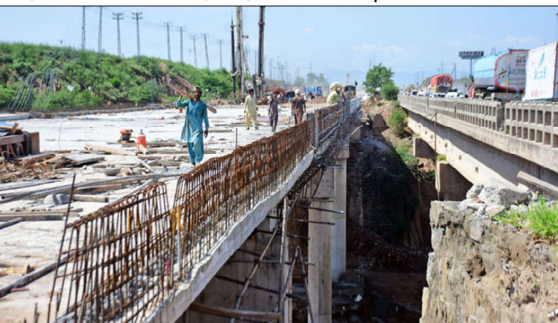
ISLAMABAD: Labourers are busy in construction work of a bridge at Islamabad highway during development work, in the Federal Capital.
