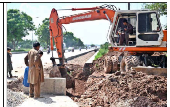
ISLAMABAD: During the expansion work of Club Road, heavy machinery is being utilized to carry out the construction and development tasks.
