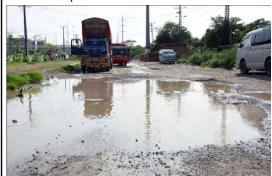
ISLAMABAD: Motorists facing difficulties due to damage service road along Karnal Sher Khan Shaheed Road after the heavy monsoon rain in the Federal Capital.
