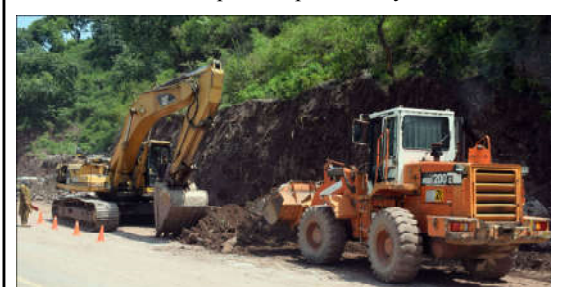
MUZAFFRABAD: Labourers are busy in construction work with the help of heavy machinery alongside a road in the city.
