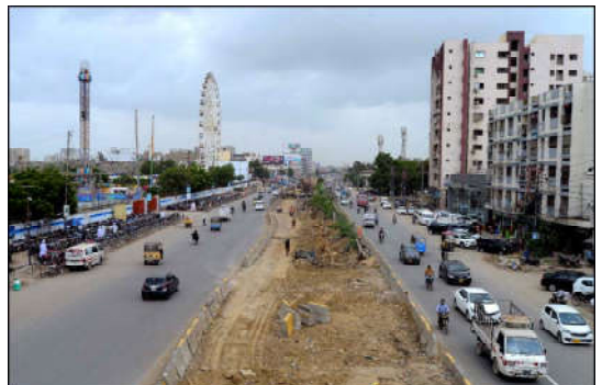
KARACHI: Construction works of new development projects is underway under the supervision of local government department, as slow pace of construction work is creating problems for commuters due to traffic jam and they demand to concerned department to complete work as soon as possible, located on University road in Karachi.
